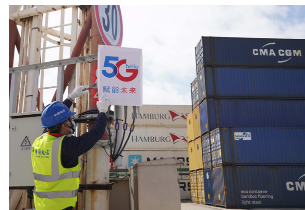
▲ China Telecom staff provisioning 5G base station for the terminal
