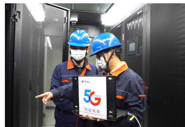
▲ Data monitoring in computer room for the Terminal
